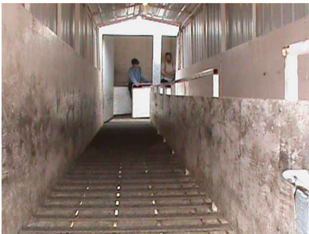
Figure 1. Covered hydraulic loading ramp with manway (looking down ramp from truck entry)
