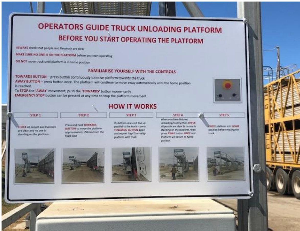
Figure 3: Signage installed at control panel of the Crate P.A.L.
