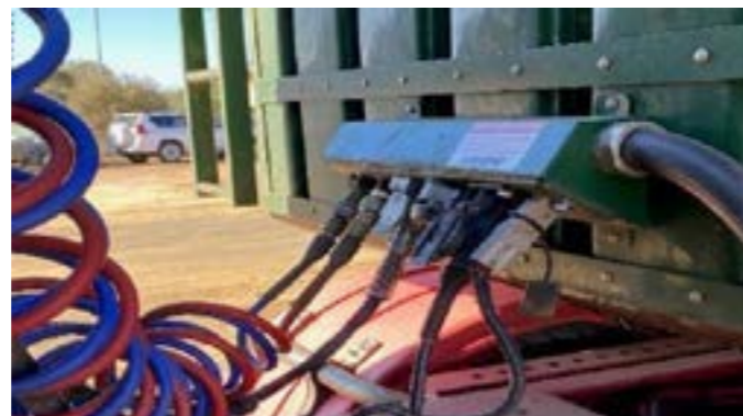
Downward-facing trailer connections to reduce debris build-up
